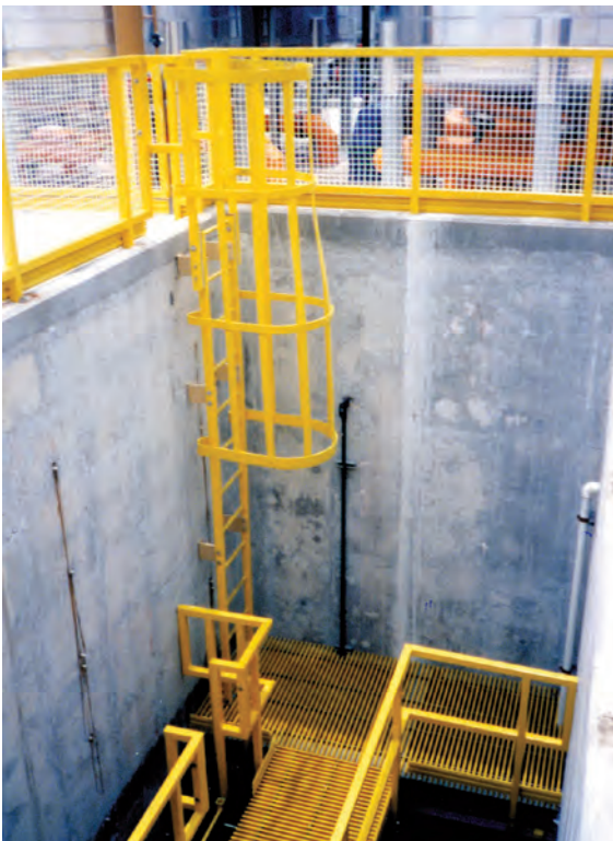
Fiberglass access ladders are used throughout the service areas of Sea World in Orlando, FL, and resist saltwater corrosion and reduce maintenance costs.
